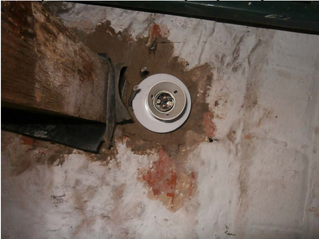
13) Exposed Live electrical conductors and light fitting a head height
